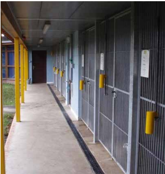
Protected external runs (showing drainage)
